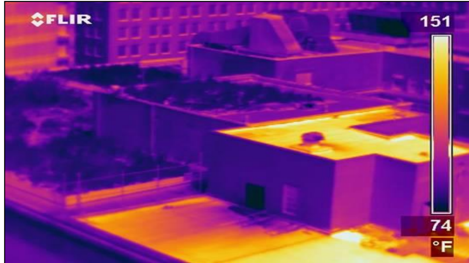
Infrared image of the roofs.
